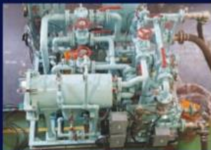
Heli fuel supply system - 1
